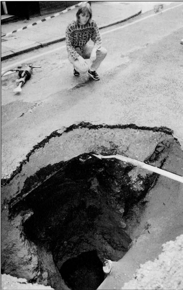
The collapse of Stanford Street very soon after it happened; most of the open hole is in soil and fill, but rock is just visible around the dark hole breaching the cave roof.
