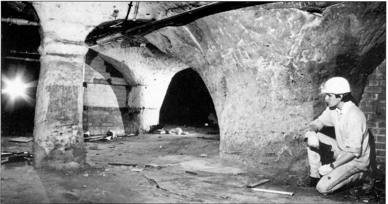
The fine columns and roof arches in the medieval undercroft cave beneath the old Pearsons department store.
